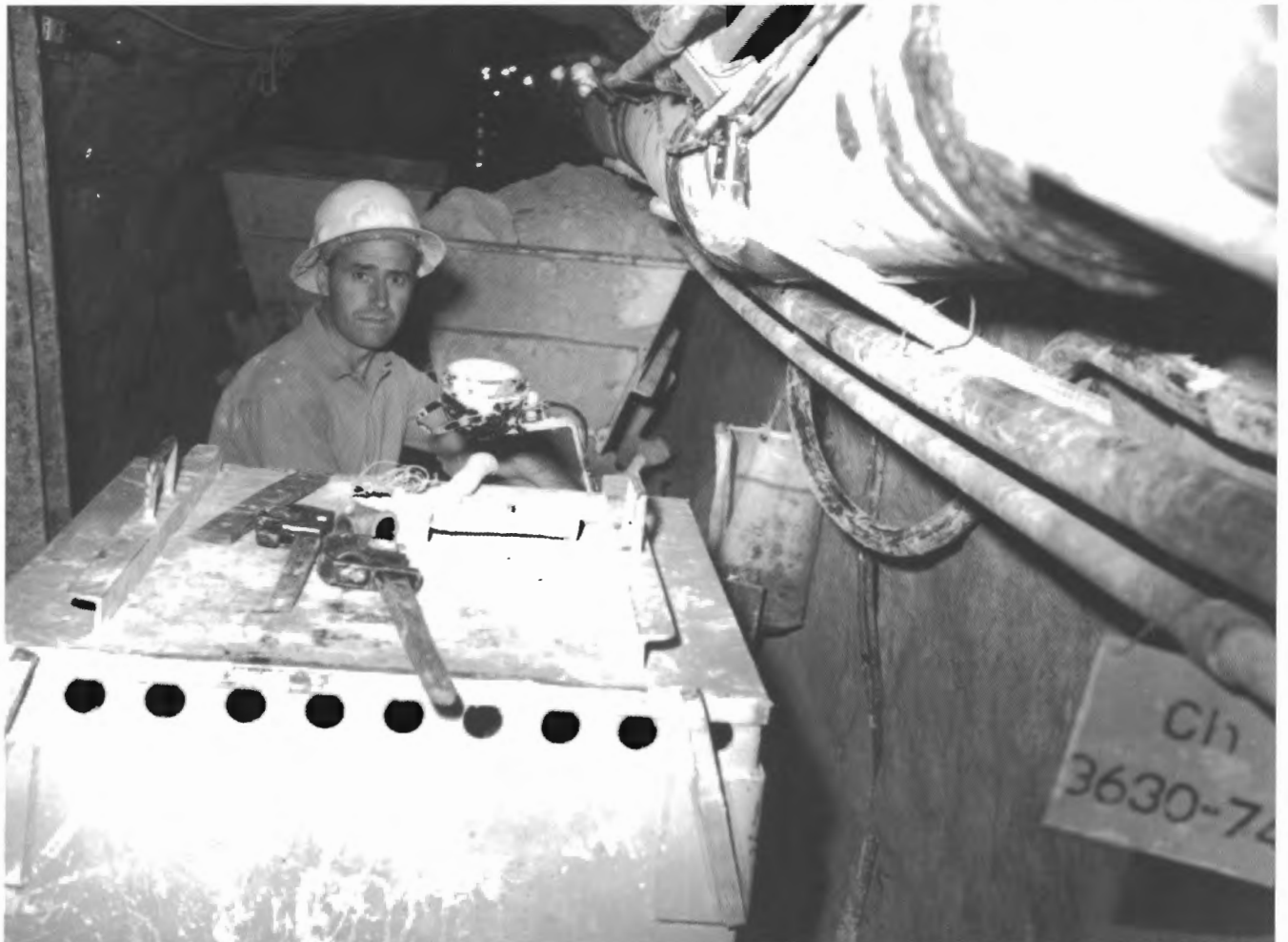
Trammer in the West Middle Harbour Sub-main showing the tightness of these small diameter tunnels, 1968
