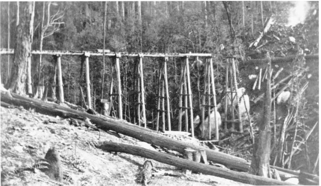
The South Cascade Bridge under construction in 1939. The bridge was built by Percy Dargie's tramway construction crew. Mrs. Dargie
