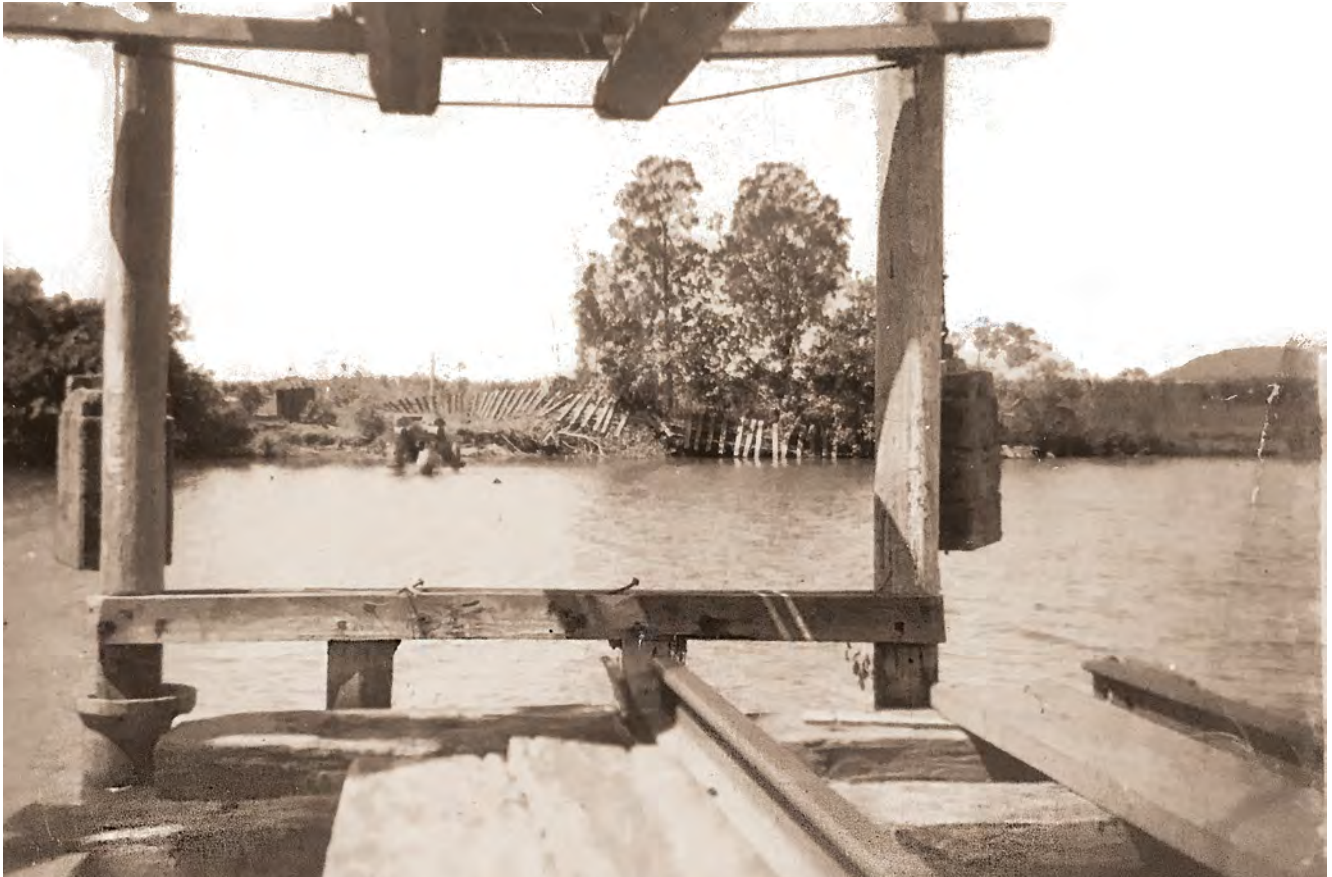
Above: Damage caused to the bridge in 1947. Note that the lift span survived but the rest of the structure has been washed away and the rail tracks holding the sleepers together are spread along the opposite bank. Photo: Clive Plater collection
