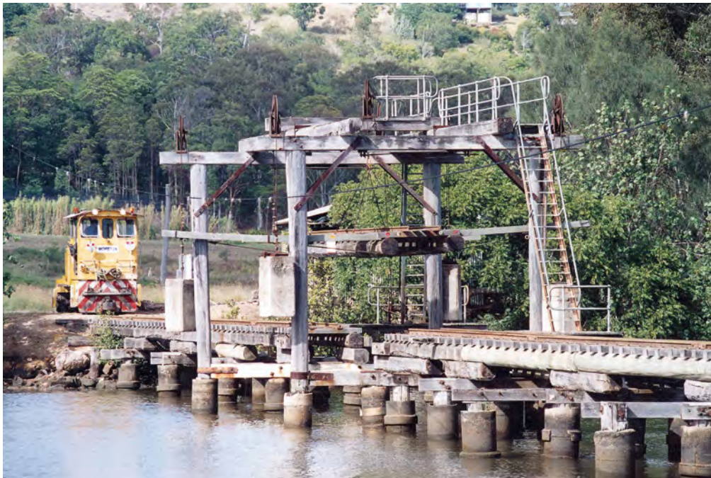
The lift section has been partially raised as locomotive Moreton looks on from the far bank on 15 August 2001. Photo: Brian Webber
