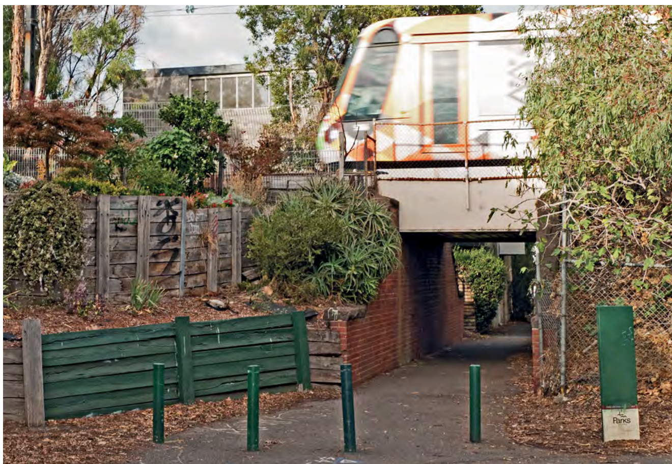
Reconstructed Military Road tramway culvert in Albert Park, April 2019. The St Kilda railway was converted to standard gauge in 1987 and is now part of Melbourne's tramway network. Photo: Colin Harvey
