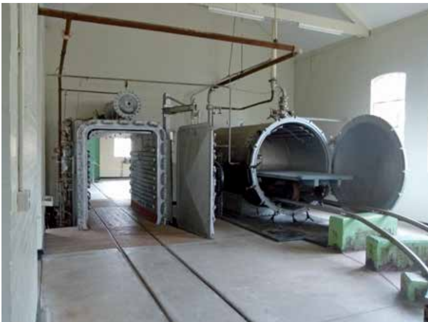
The two autoclaves. A small wooden-framed trolley sits inside the circular unit Photo: Andrew Forbes
