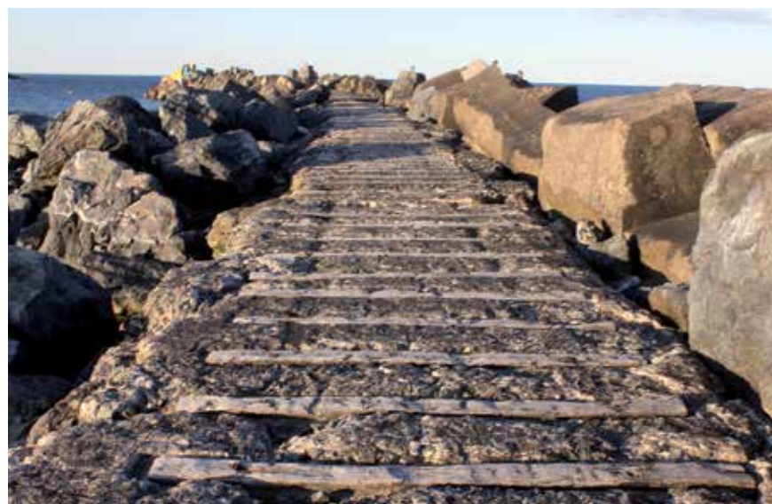
The remains of the Coffs Harbour breakwater tramway, last used in 1974 and soon to be covered forever as reconstruction works raise the wall level, seen on 25 August 2012
