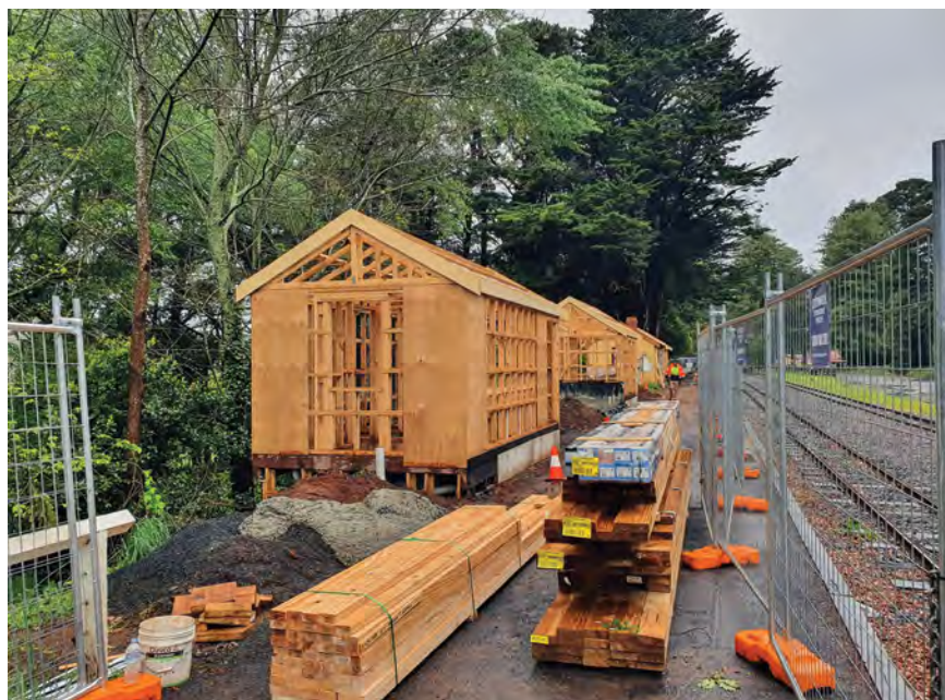
New building works at the Gembrook station on the Puffing Billy Railway in November 2022. Both photos: Andrew Rayment
