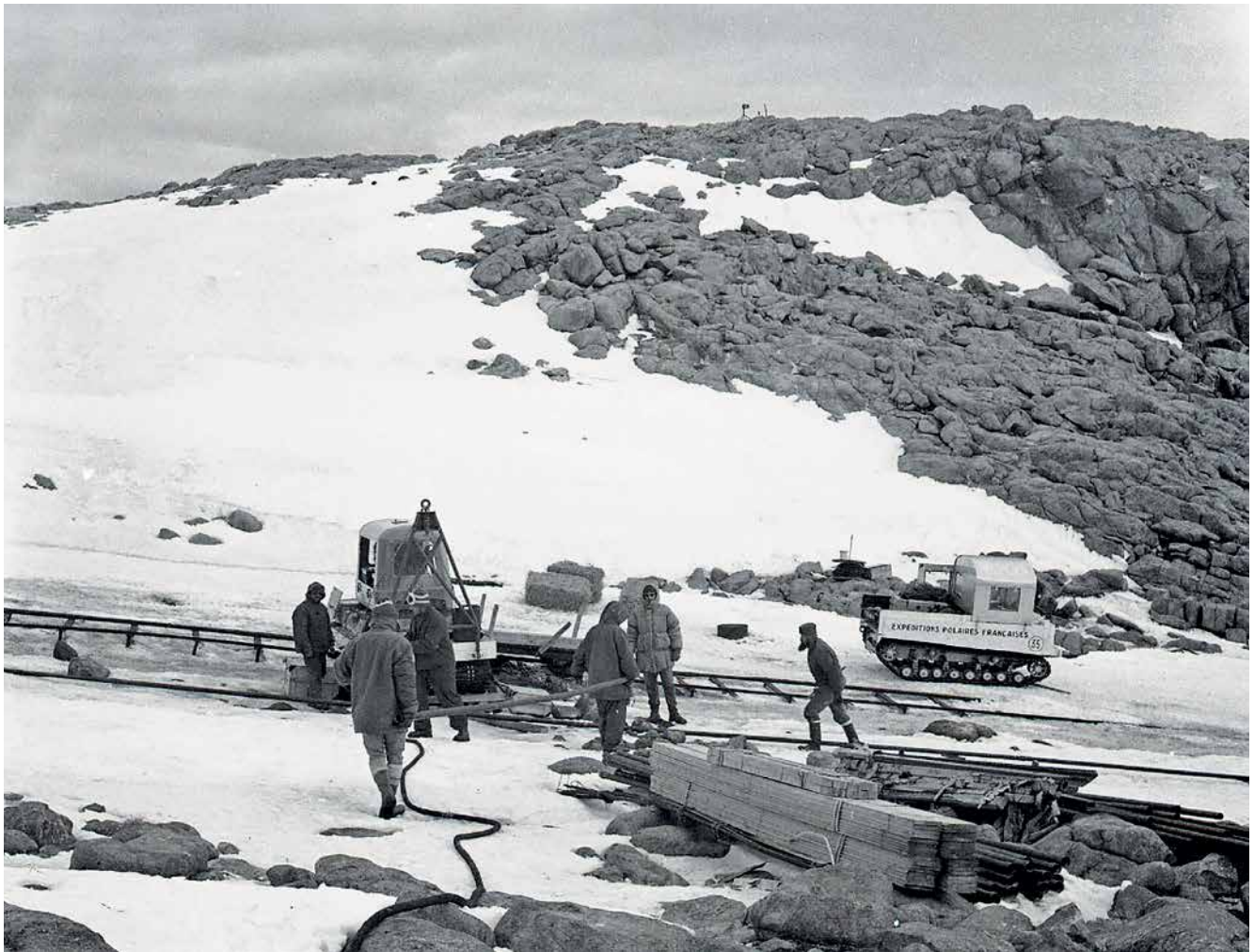
The narrow-gauge incline railway used to move materials and supplies to the centre of the base, 1958. There seems to have been a crisis – a derailment maybe, or are they laying a pipeline under the railway? The track is steel rails on steel sleepers that have vertical anchors for additional holding.
