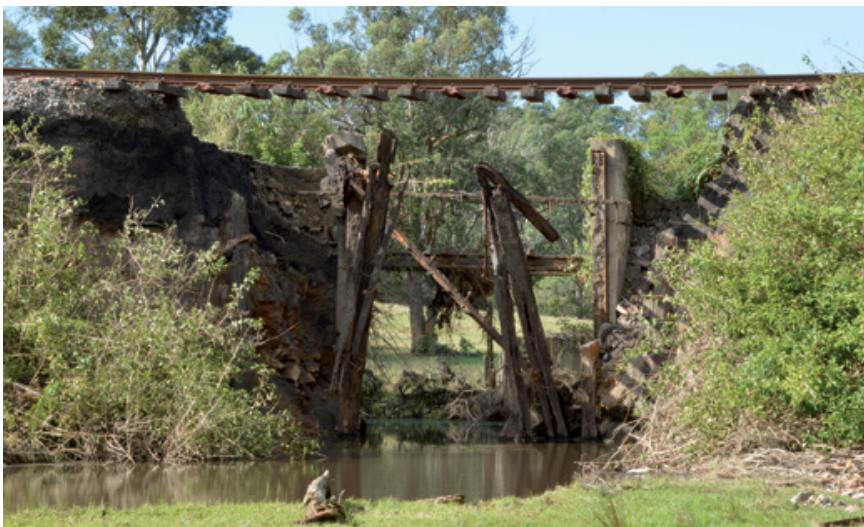
During the storm of 20 and 21 April, this washaway at 5.05 kilometres on the South Maitland Railway exposed the timber supports of the former viaduct and underpass which were buried in situ in the 1970s. Photo: James Knight
