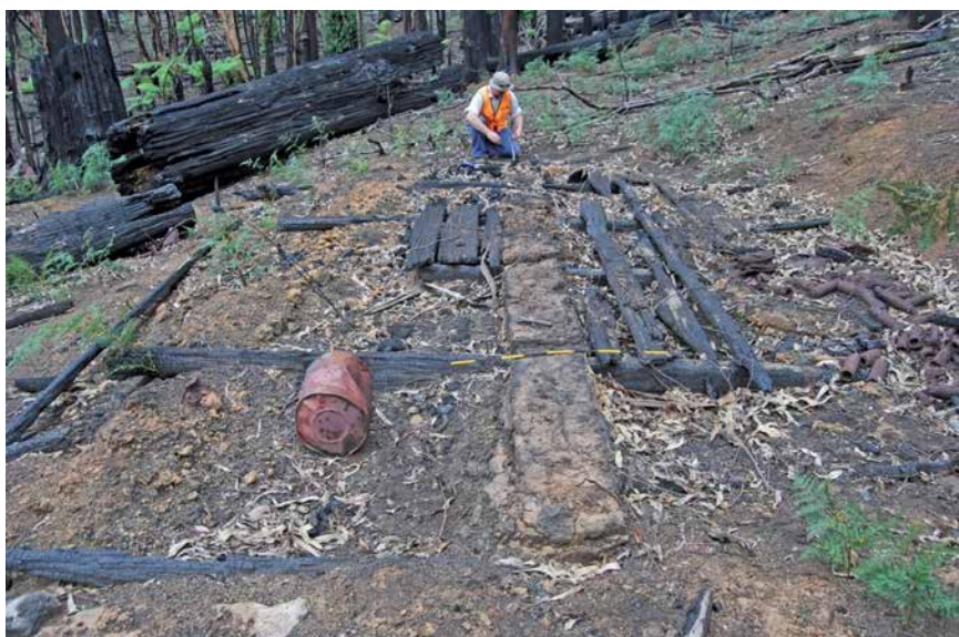
C: Scott Gould examines the foundations of the crawler-tractor servicing shed at the 'S' Creek mill. Note the worn and abandoned track rollers on the right of frame. Photo: Peter Evans
