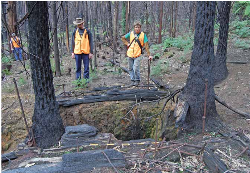
A: The foundations of the breaking-down bench at the 'S' Creek sawmill. From left to right (resplendent in the LRRSA 2009 post-fire survey hi-vis vests), Scott Gould, Stuart Thyer and Stefan Rebgetz. Photo: Peter Evans
