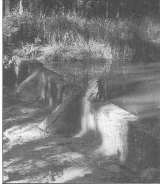
A small concrete dam built by Pines & Hardwoods below the Apple Tree brush line. It held water for the steam log haulers and, in emergency, the locomotives.
