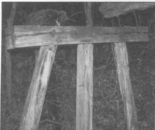
Remains of a trestle bridge 3km north of the mill in 1991. Note the characteristic triple pile arrangement, topped by a double horizontal corbels bolted through the tops of the piles. Bridge girders rested directed on the corbels.
