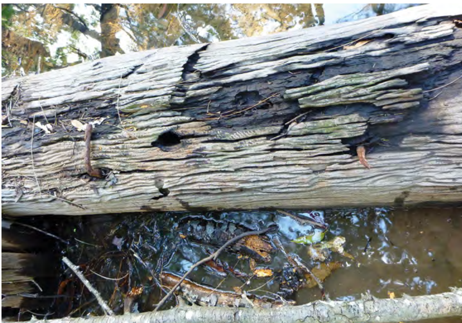
Iron spike in a bridge stringer. Photo: Ian Barnes
