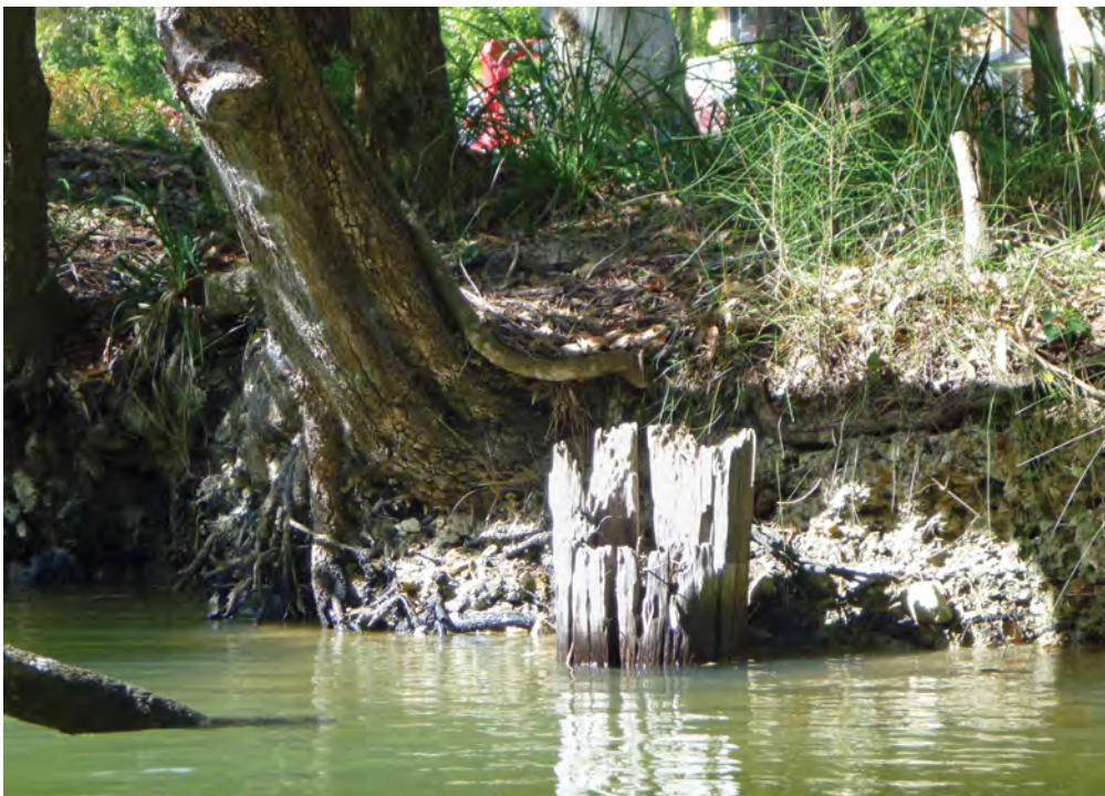
At the southern bank of Poundyard Creek is a solitary bridge pile and a shallow box cut approach. Photo: Ian Barnes
