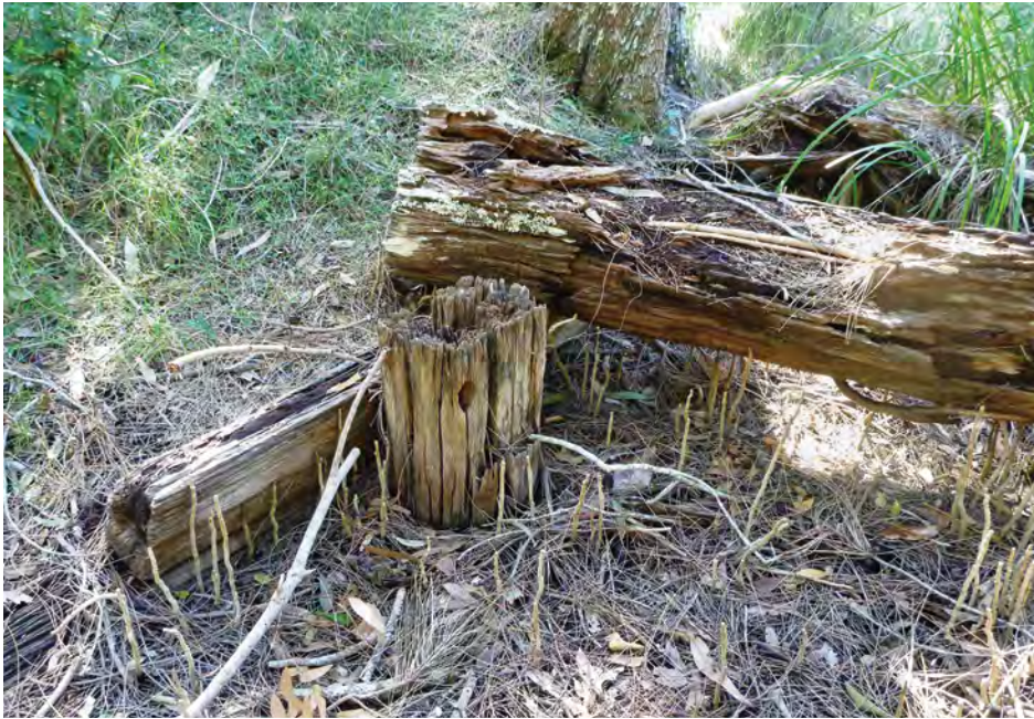
At the northern bank of Poundyard Creek are more substantial abutment remains. Photo: Ian Barnes
