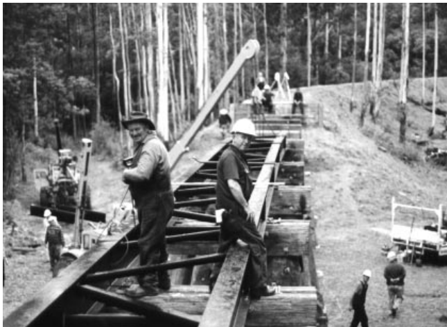
On 21 February, PBR identities Dave Conlan and Don Marshall take a breather as construction work continues on Bridge No.9, which will carry the Gembrook extension over Cockatoo Creek Photo: Bill Hanks
